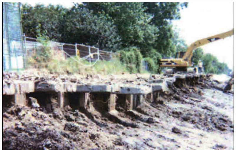
FIGURE 5: EQUIPMENT SUPPORT MOVED DOWNWARD AND OUTWARD DURING DRY SLOPE CONSTRUCTION
