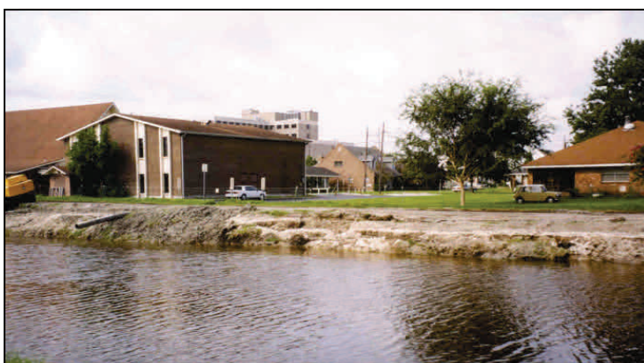
FIGURE 3: FAILED CANAL BANK DURING CANAL BOTTOM CONSTRUCTION
