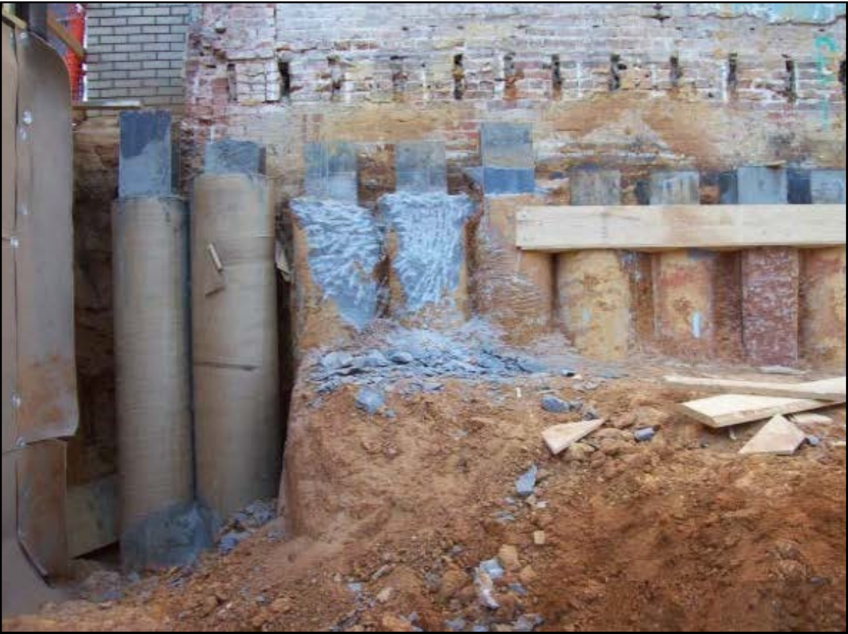
FIGURE 3: SUCCESSFULLY INSTALLED MODIFIED SECANT WALL CONSISTING OF STIFF CONCRETE SHAFTS THAT PROTECTED IMMEDIATE EXISTING BUILDINGS
