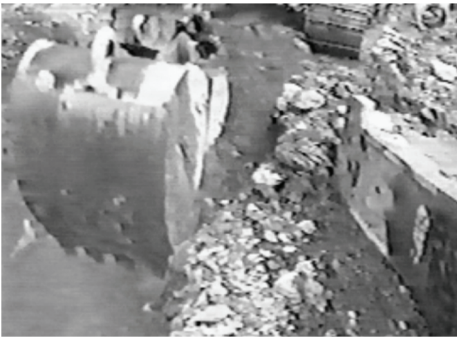
FIGURE 2 PICTURE SHOWS CONTRACTOR USING A 300 HP EXCAVATOR FOR RIPPING ROCK. CONTRACT REQUIRED 160 HP EXCAVATOR TO DETERMINE HARD EXCAVATION QUANTITIES
