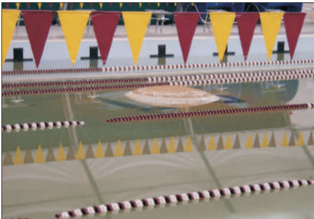
FIGURE 1 VERY LARGE BUBBLE IN THE FLOOR LINER WHICH GREW OUT OF THE WATER DURING THE OPERATION OF THE POOL
