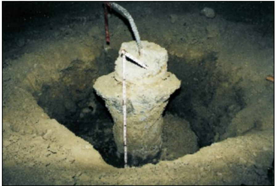
FIGURE 1 TYPICAL PICTURE SHOWING THE MUSHROOMING OF THE PIER TOP
