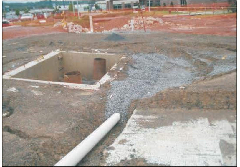
FIGURE 1: PICTURE SHOWING SAG SUBSIDENCE WHICH FORMED DURING CONSTRUCTION AND ENCOMPASSED AN ELEVATOR PIT
