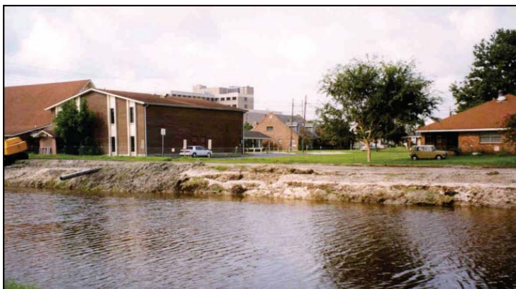
FIGURE 3: FAILED CANAL BANK DURING CANAL
