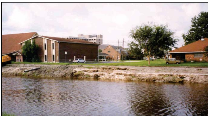
FIGURE 3: FAILED CANAL BANK DURING CANAL
