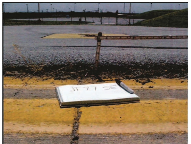
FIGURE 1: DIFFERENTIAL HEAVE OF 1.3 IN. FROM SUBGRADE SWELLING BETWEEN THE TAXIWAY
