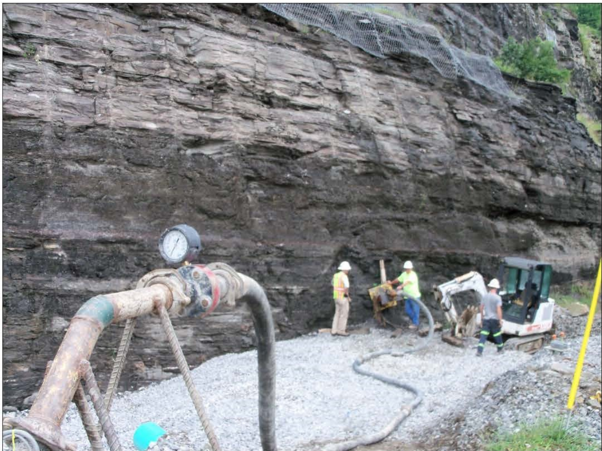
FIGURE 3: GROUT INJECTION WITH PRESSURE INTO THE MINE OPENING FILLED WITH CAVE MATERIAL ALONG THE ROCK CUT.
