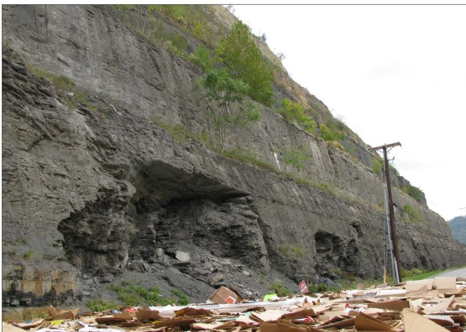
FIGURE 2: MINE OPENINGS IN 400 FT. HIGH ROCK CUT. MINE ROOF CAVED UPWARD OVER TIME.
