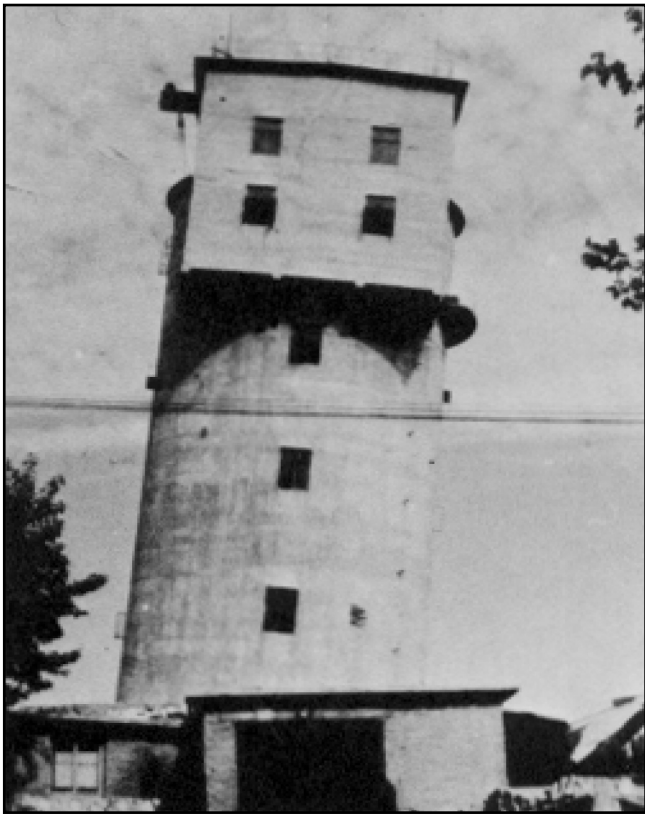
FIGURE 2 TILTED VENTILATION TOWER AT THE TANGSHAN COAL MINE FROM THE GREAT TANGSHAN EARTHQUAKE (CALIFORNIA INSTITUTE OF TECHNOLOGY, 2002)
