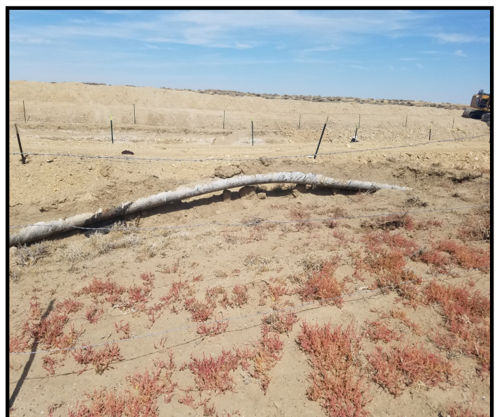
FIGURE 2 UPHEAVAL BUCKLING OF A PIPELINE FROM LAND SUBSIDENCE FROM MINING
