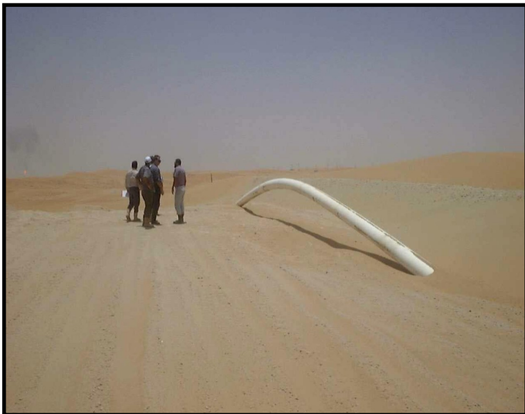
FIGURE 1 UPHEAVAL BUCKLING OF A PIPELINE IN DESERT TERRAIN (TR ENGINEERING CONSULTANCY)
