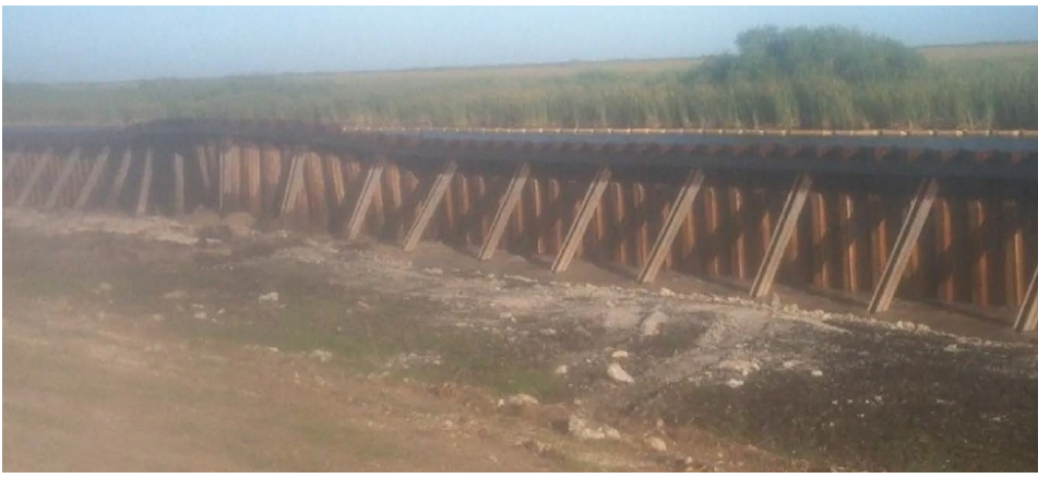
FIGURE 2 VIDEO OF ONGOING BREACH OF THE COFFERDAM DUE TO UNDERSEEPAGE
