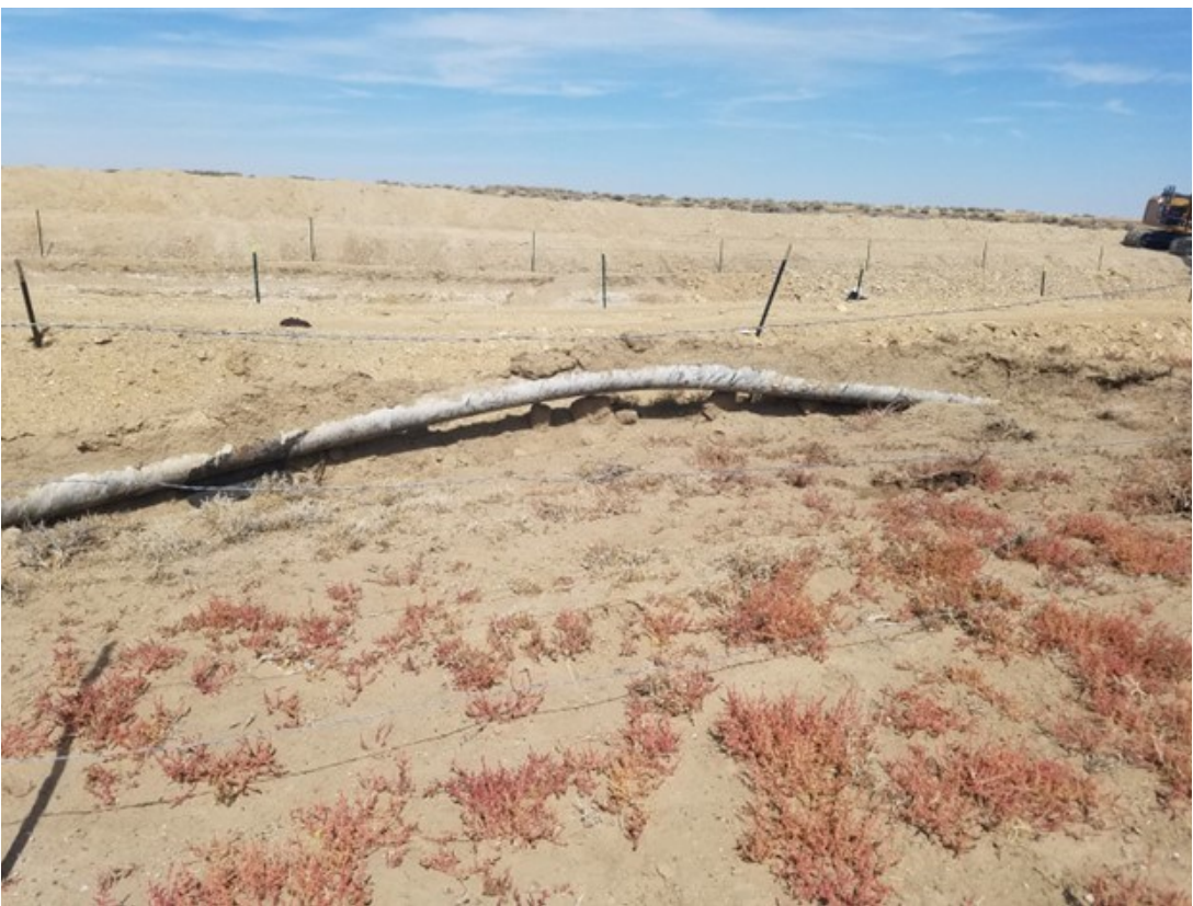
FIGURE 2 EXAMPLE OF UPHEAVAL BOWING OF A GAS TRANSMISSION FROM MINE SUBSIDENCE
