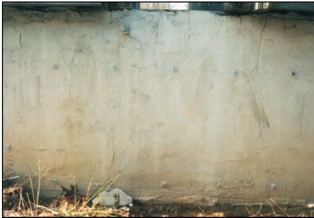
FIGURE 4 PHOTOGRAPH OF FACE OF FIBER-CEMENT COATING ONE YEAR AFTER APPLICATION
