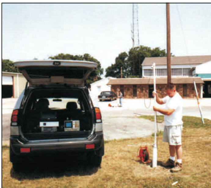
FIGURE 1 MEA BOREHOLE RADAR SYSTEM: ANTENNAS BEING LOWERED INTO BORINGS IN ORDER TO CONDUCT A CROSS-HOLE SURVEY
